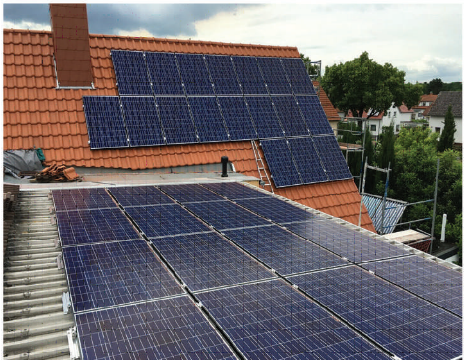
Mannheim 10kWp rooftop solar system, Germany
